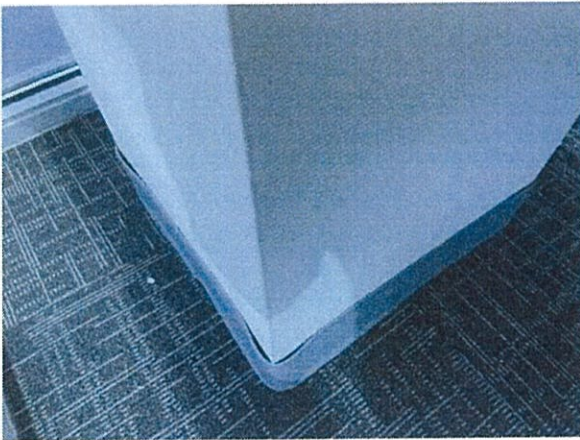
1. Rubber base at columns not properly Installed.
