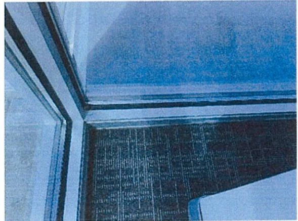
2. Carpet not properly cut; concrete gap can be seen.
